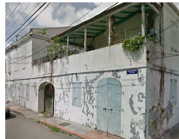
Example of the disrepair facing many buildings in the Territory.
